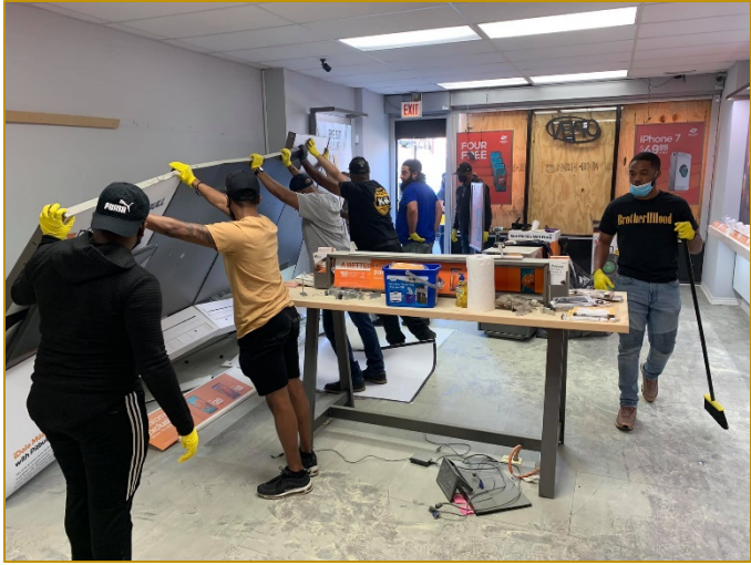
Men of Alpha assisting in the re-construction of Bro. James Leuthe Boost Mobile store after the Looting in Chicago.
